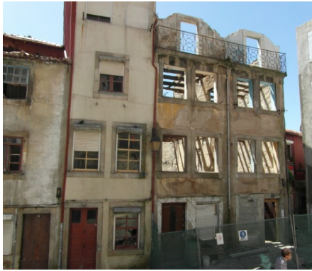
Fig. 1 – Undergoing rehabilitation under the resettlement program, recovering some old buildings which were totally destroyed.
